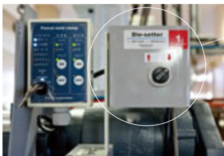
Die setter operation panel
